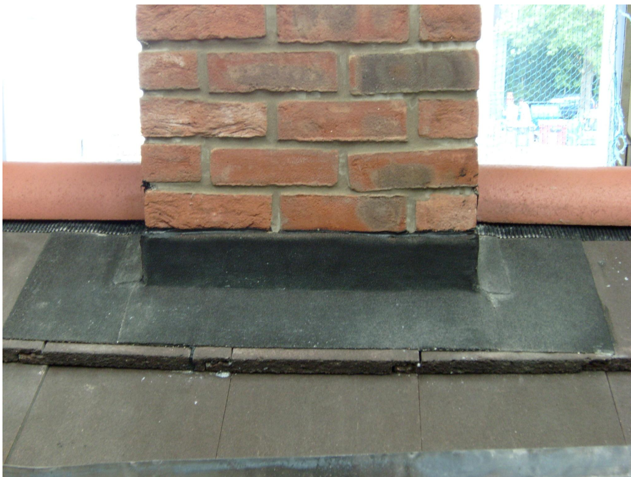
Figure A1 side 2 showing flashing after completed test programme 45m/s (101mph)
